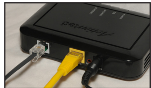
NOTE: MAKE SURE ALL DEVICES WITH THE SAME PHONE NUMBERS AS YOUR DSL LINE HAVE FILTERS.
